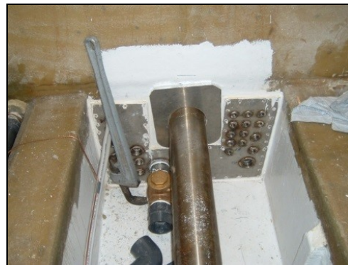
Figure 3.0(b)(ii): Arrangements to ensure the watertightness of piping passing through a bulkhead in a fishing vessel. (Courtesy of J.G. Personal collection)
