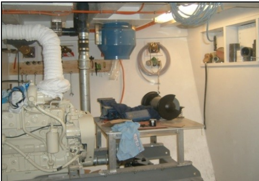
Figure 3.0(b)(i): Below deck machinery in the engine room of a fishing vessel. (Courtesy of J.G. Personal collection)
